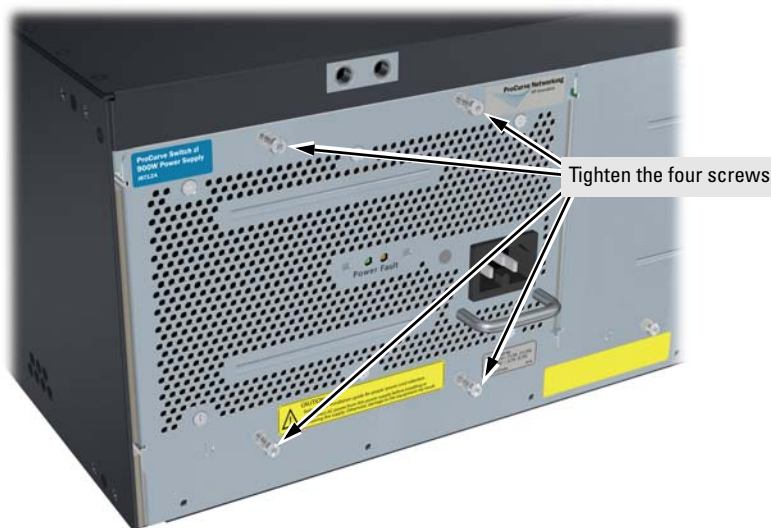
Figure 4. Fully installed power supply
